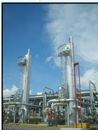
Figura 2.2 Torres contactoras T-1150/1160.
