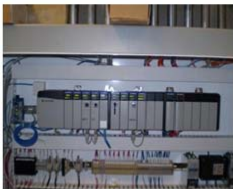
Figura 3.4: Allen Bradley PLC.
